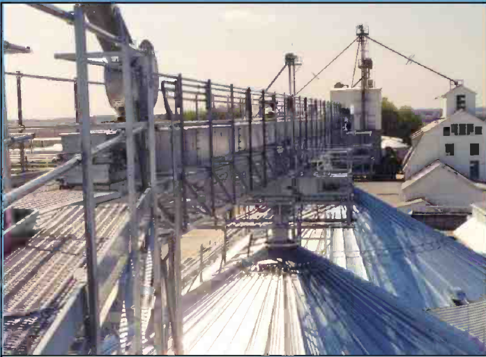
Conveyor support with conveyor and manwalk in foreground
