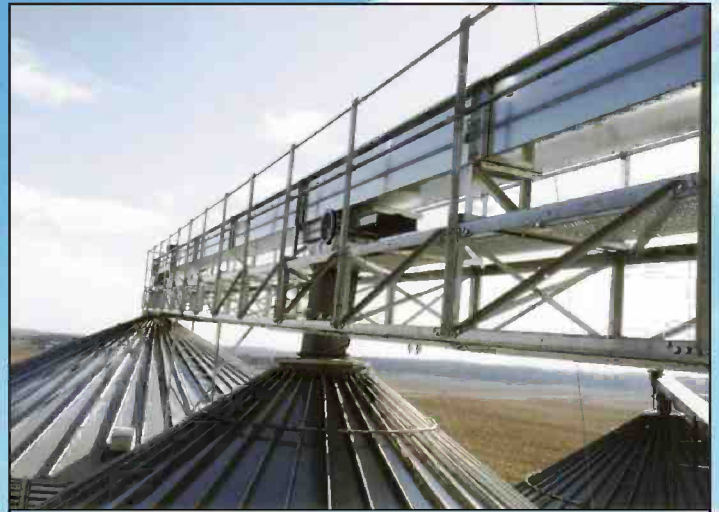
24" tall lower bridge truss with diagonal braces on sides, top and bottom cross bracing
