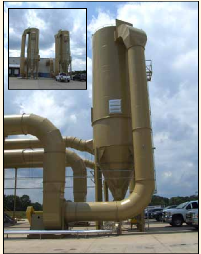
One of two negative system backward curve fans with a medium pressure cleaning baghouse filter.
