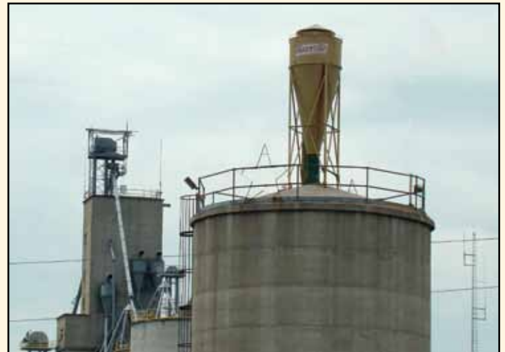
In this application, the cyclone is being used as a silo receiver cone at a sawmill.
