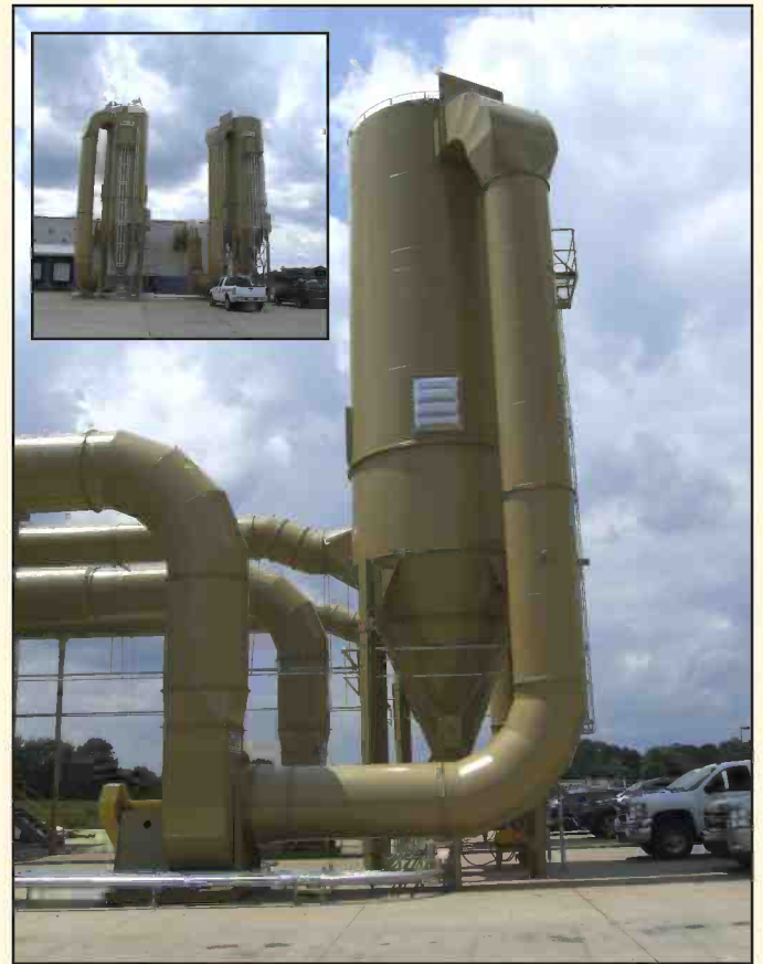
One of two negative system backward curve fans with a medium pressure cleaning baghouse filter.
