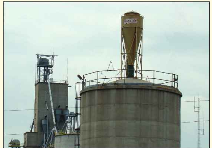
In this application, the cyclone is being used as a silo receiver cone at a sawmill.
